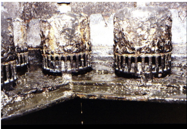
FIGURE 3-3 Sour corrosion of bubble caps.
