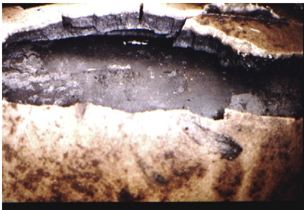
FIGURE 3-13 Salt fouling fire tube. (Courtesy of Gly-Tech)
