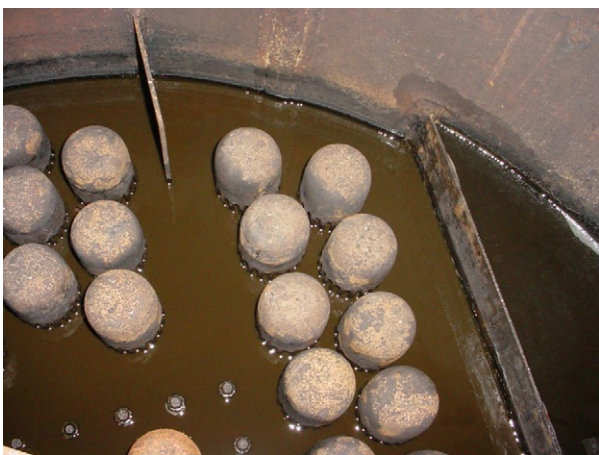
FIGURE 2-37 Bubble cap tray inside the contactor tower.
