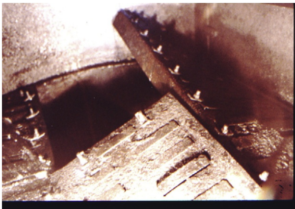
FIGURE 3-16 Tray damage due to compressor failure.
