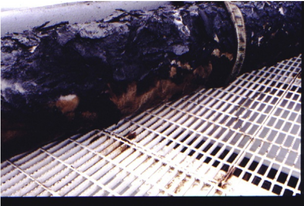
FIGURE 3-29 Decomposed glycol with fire-tube burnout.
