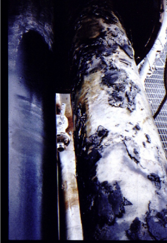
FIGURE 3-27 Decomposed glycol on reboiler fire tube. (Courtesy of Gly-Tech)
