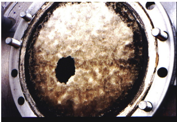
FIGURE 3-12 Salt deposited in interior of reboiler. (Courtesy of Gly-Tech)
