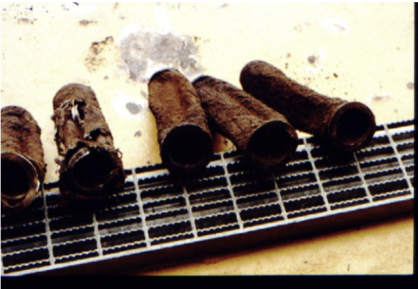
FIGURE 3-34 Filter collapsed due to high-pressure drop.
