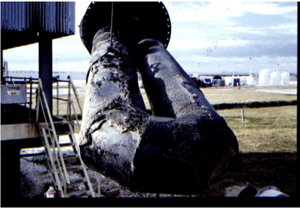
FIGURE 3-26 Decomposed glycol on reboiler fire tube.
